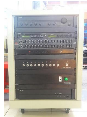
Public Address System (PA System)
