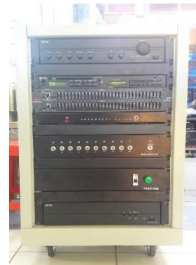
Public Address System (PA System)
