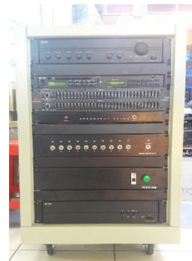
Public Address System (PA System)
