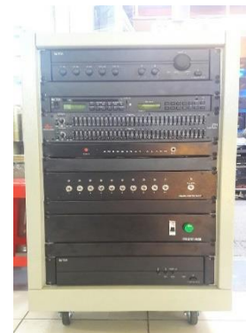
Public Address System (PA System)
