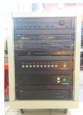
Public Address System (PA System)
