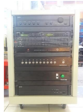
Public Address System (PA System)
